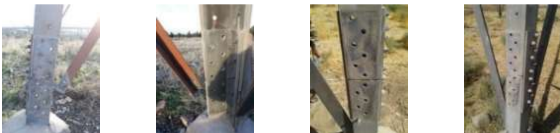
Fig. 1. Theft of the bolts of the connected members in the leg of the power transmission towers
