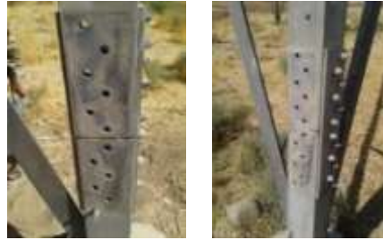
Figure 1- Theft of the bolts of the connected members in the leg of the power transmission towers
