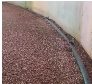
Fig. 2. Porous tube installed in the bend
