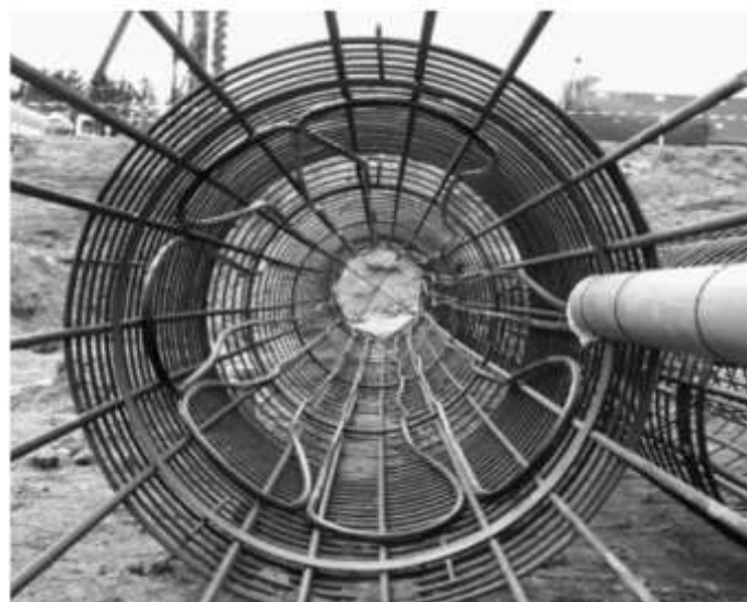
Fig. 1. Absorber pipes fitted to the reinforcement cage of a large-diameter bored energy pile (Brandl, 2006)
